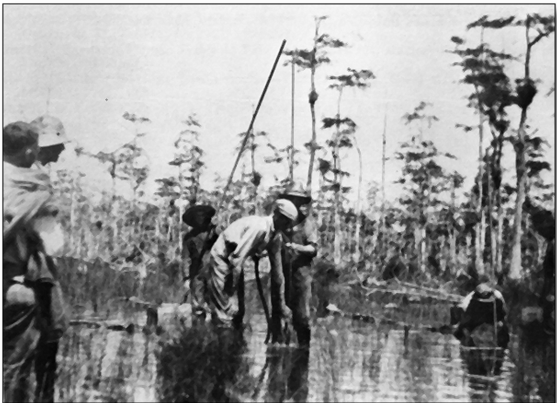
Dynamite Setters—Some of the men who set dynamite by tamping the sticks into pipes in the rock base two to five feet below the surface of the water line
