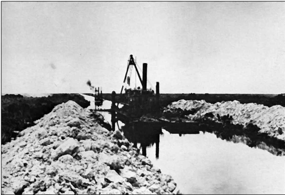
Walking Dredge— Unique dredge used exploded aggregate to create both a canal and a road bed. The dredge moved forward by jacking itself up and extending its bucket to skid forward by eight to ten feet. This “hop-a-long” dredge made the Tamiami Trail possible
